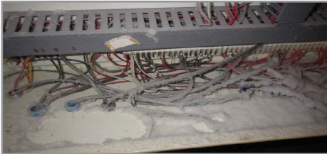
▲ Control panel before decontamination
