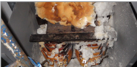
▲ Transformer with the burnt cotton before decontamination
