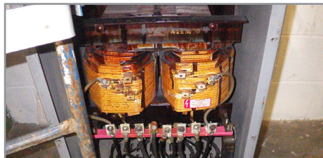
▲ Transformer with the burnt cotton after decontamination
