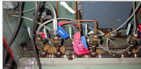
▲ Backside of line R-4 operator's station after decontamination
