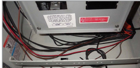
▲ Motor control center (MCC) circuit breaker panel after decontamination
