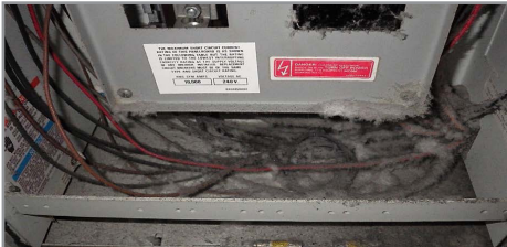
▲ Motor control center (MCC) circuit breaker panel before decontamination
